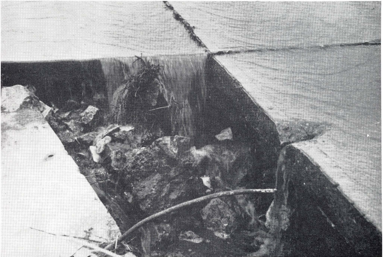
Heavy rains resulted in this damage to the spillway apron in the year 1940. Such occurrences pose a problem of constant maintenance at the State Lakes in Kansas.
